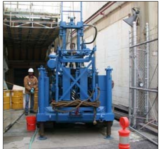
Drill used to install monitoring wells at Indian Point. Ground penetrating radar is used to ensure that the drill will not intercept buried service lines. Then a vacuum drill is used for the first 6-8 feet followed by a diamond bit drill for the deeper depths.
