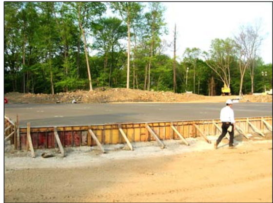
Fuel from Indian Point's spent fuel storage pools will be loaded into shielded casks and placed on this storage pad. The picture shows the pad under construction.
